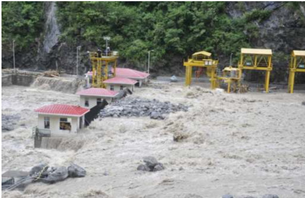
Damaged Vishnuprayag Dam in Uttarakhand floods of June 2013. Source: MATU Jansangathan
