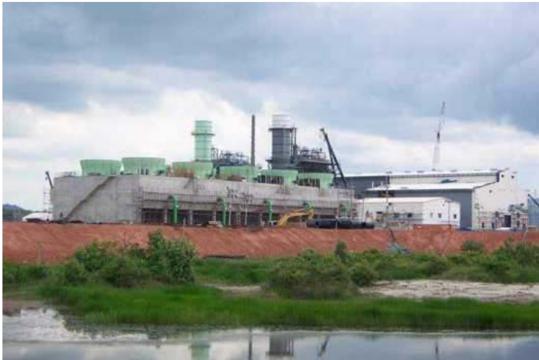
The EGAT electricity generating station at the end of the pipeline.
